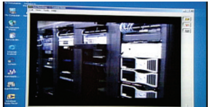
Using category 6 cabling
